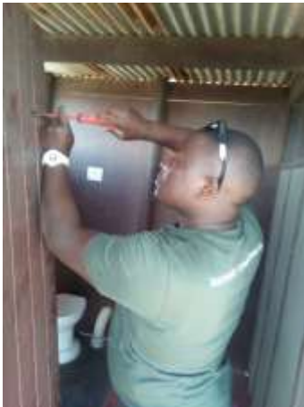
Figure 29 Lamla Sigenu repaired the door of the public ablutions at Blaauwberg Hill
